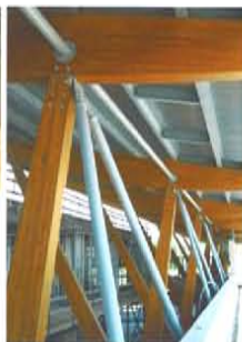
Photos courtesy of Bunting Coody Architects
